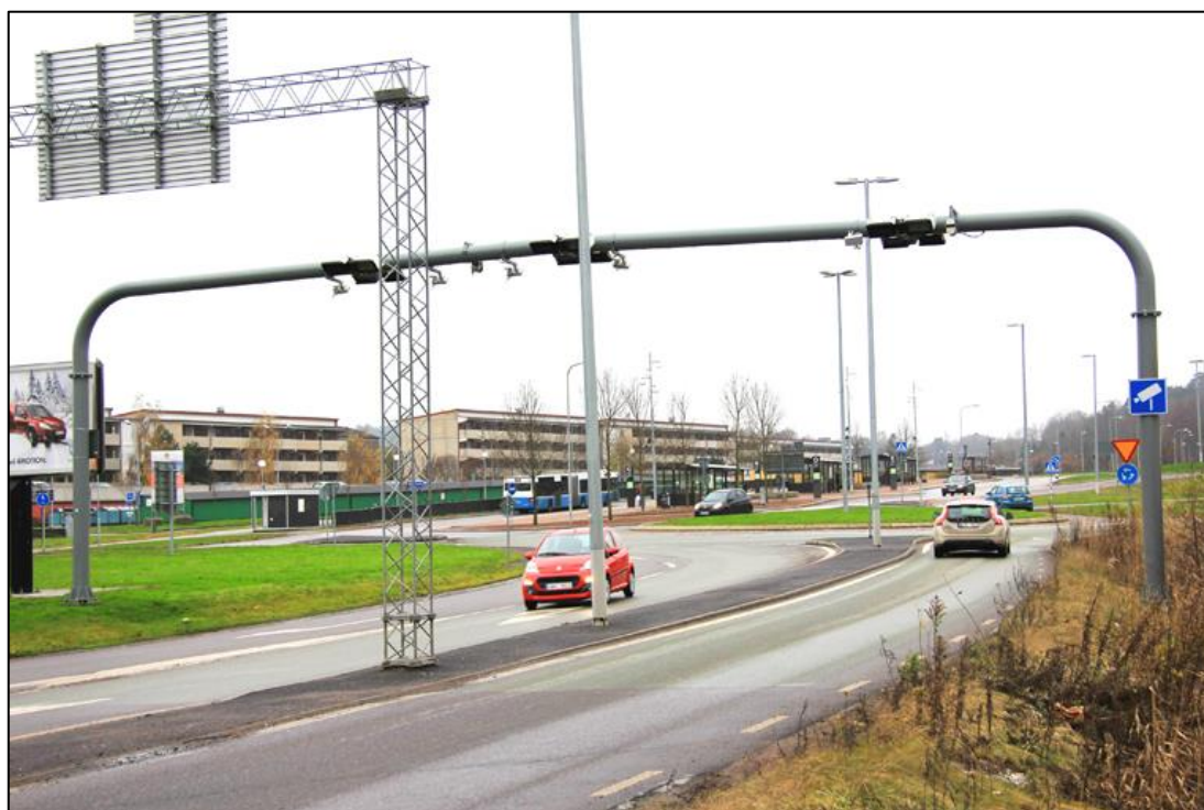
Figure 31 - Gothenburg ANPR gantry
